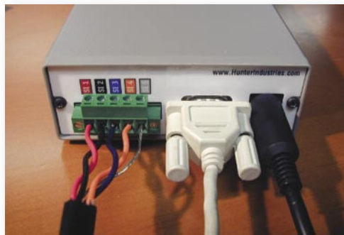
Figure 9: CCC GCBL wiring
